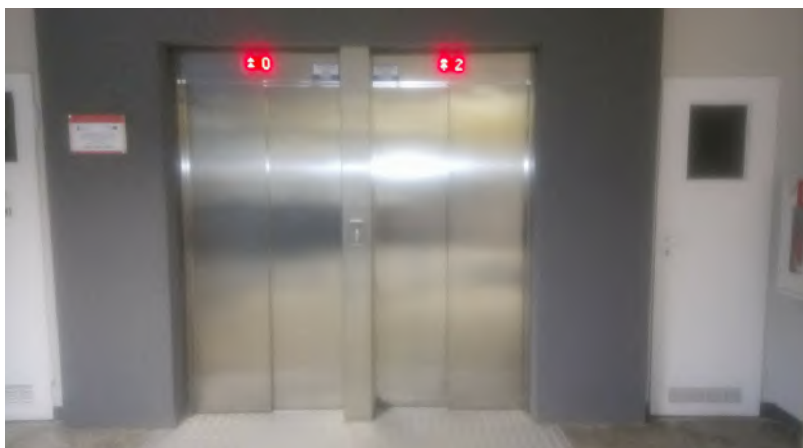
Fig. 2. Lifts of the "B" building of the Gdańsk University of Technology after renovation
